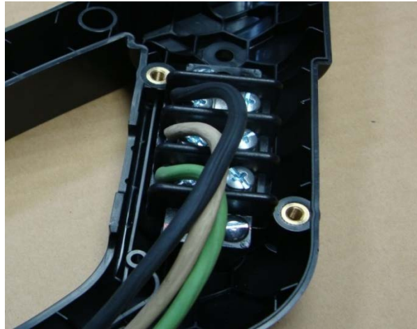
Fig.6-6 Terminal Block Wiring
